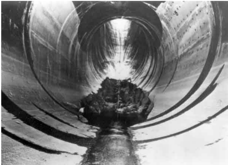
Figure 6.5. Cavitation damage to the concrete wall of the 15.2 m diameter Arizona spillway at the Hoover Dam. The hole is 35 m long, 9 m wide and 13.7 m deep. Reproduced from Warnock (1945).
